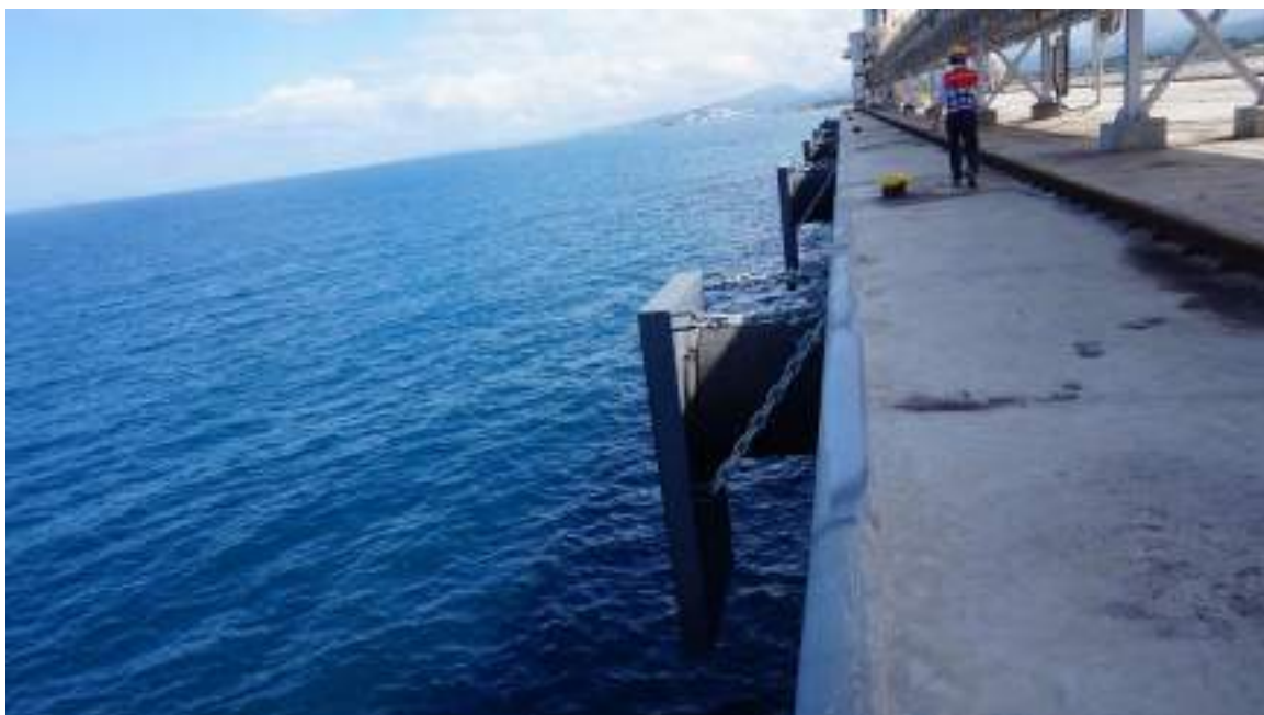
TOLEDO POWER PLANT JETTY, TOLEDO CITY, CEBU HICOR CELL TYPE FENDER
